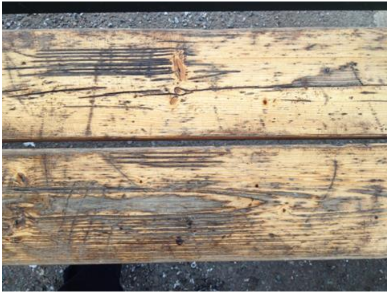
Degraded clear coated wood in outdoor use
