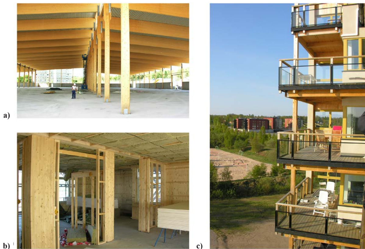
Figure 3.3: Examples of members subjected to compression forces. a) Columns in a timber frame, b) studs in a multi-storey timber framed building, c) external columns.
